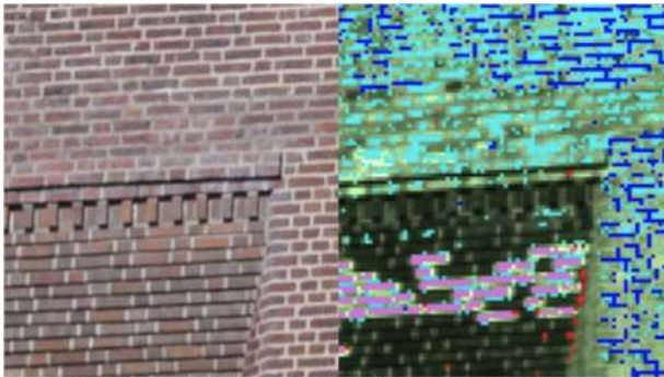
A photograph of a brick wall on the left appears fairly uniform in composition. However, the hyperspectral image on the right reveals there is a section of very different bricks, possibly due to a change in a different source of bricks in the brick's composition.
